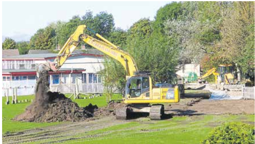
Our roving 'Reader Photographer' John Williamson was on the spot again, when work began on the new Vane Road School. If you have an interesting town photo please send it in to: syd@newtonnews.co.uk
